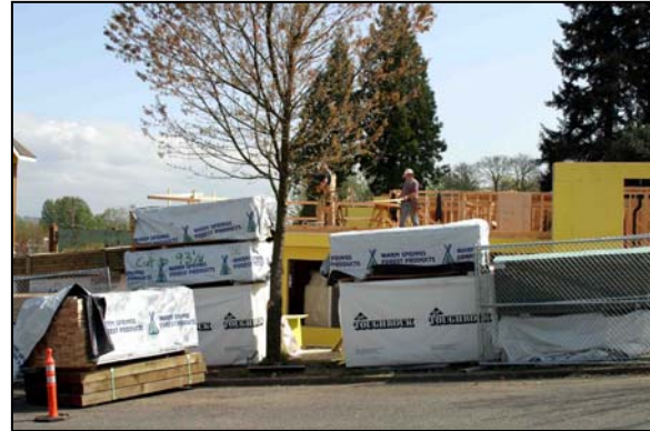
FSC-certified Warm Springs lumber and Roseburg plywood arrives at the Fenwick construction site.
